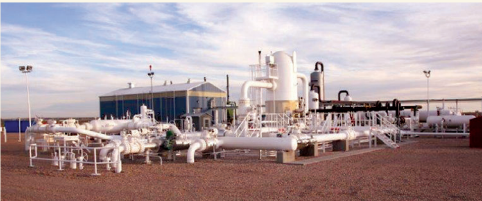
Natural gas compressor station.
