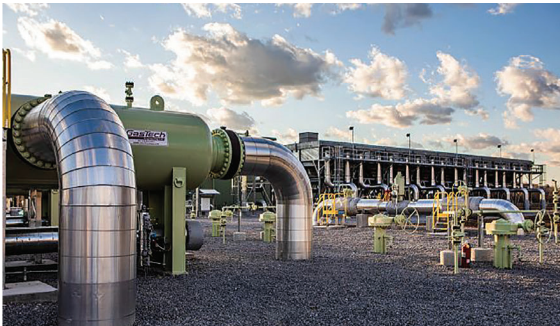
Gas transmission compressor station. (Source: TC Energy)
