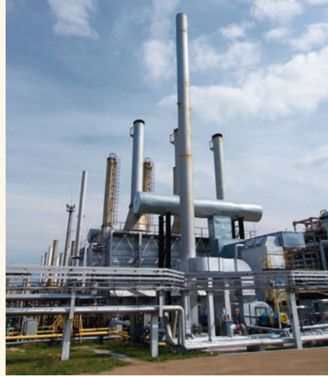
Natural gas processing facility.
